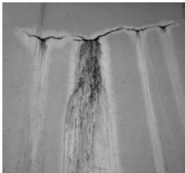
Surface peeling: Cracks that appeared on the left side of the Penchala Tunnel.
