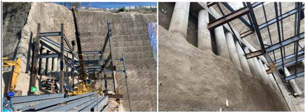
Figure 13. Continuation of the placement of dowels fastened with tie beams up to the crowning beam and piles.
