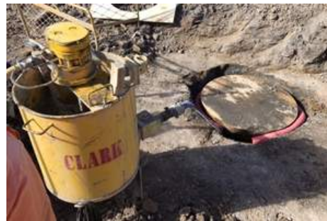
(c) A high-strength grout is mixed and placed into the annulus via a lay-flat grout tube
