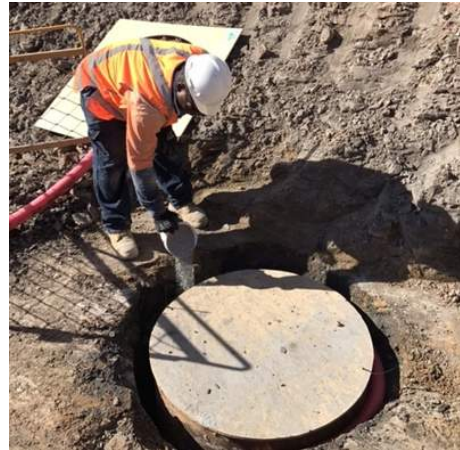
(b) The pile hole is protected with a plywood cap and the casing is fixed in place with a nominal 500mm grout plug at the base of the annulus.
