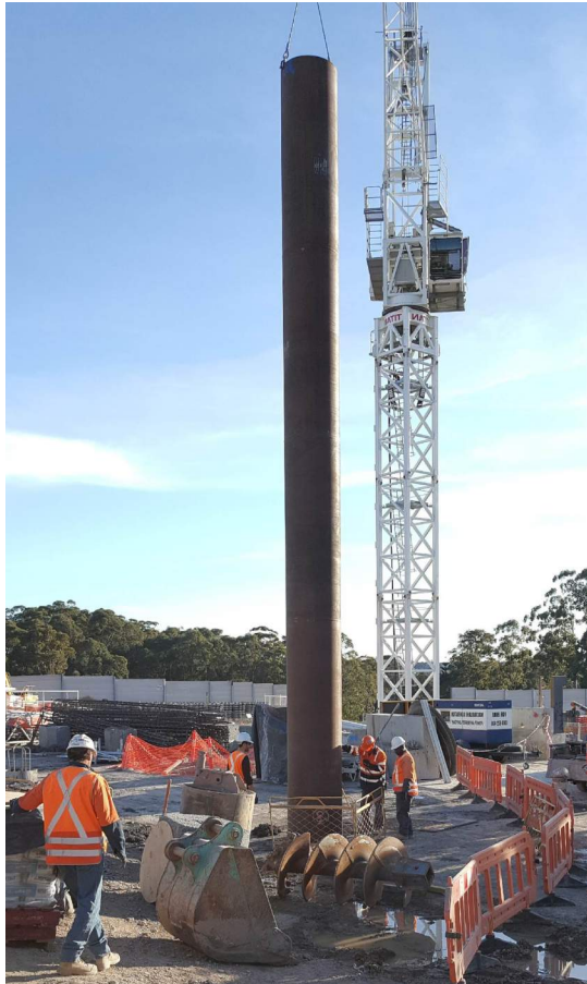
(a) The 14.35m long permanent steel casing for a pile is craned into the oversized 1050mm diameter hole by the tower crane
