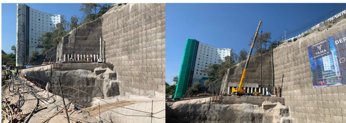
a) Continuation of excavation in central core and construction of deep piles up to 45m according to project.
